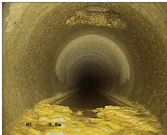
Photo: 8_2A, Media No.: 010208_1, 00:00:00 11.4FT, Tap Break-In Active, at 12 o'clock, 5", within 8 inches of joint: YES
