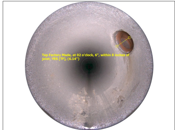
Photo: 7_7B, Media No.: 010208_1 177.99FT, Tap Factory Made, at 02 o'clock, 6", within 8 inches of joint: YES
