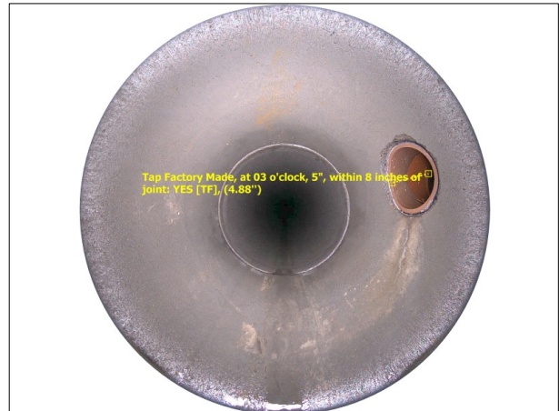
Photo: 7_3B, Media No.: 010208_1 90.59FT, Tap Factory Made, at 03 o'clock, 5", within 8 inches of joint: YES
