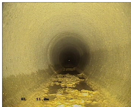
Photo: 8_4A, Media No.: 010208_1, 00:03:27 33FT, Deposits Settled Other, 5 %of cross sectional area, from 05 to 07 o'clock, , within 8 inches of joint: NO / deposits SOFT
