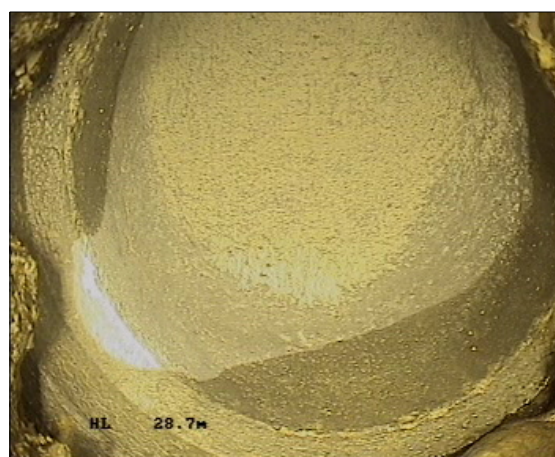
Photo: 8_6B, Media No.: 010208_1, 00:07:46 85.5FT, Tap Break-In Active, at 11 o'clock, 5", within 8 inches of joint: YES
