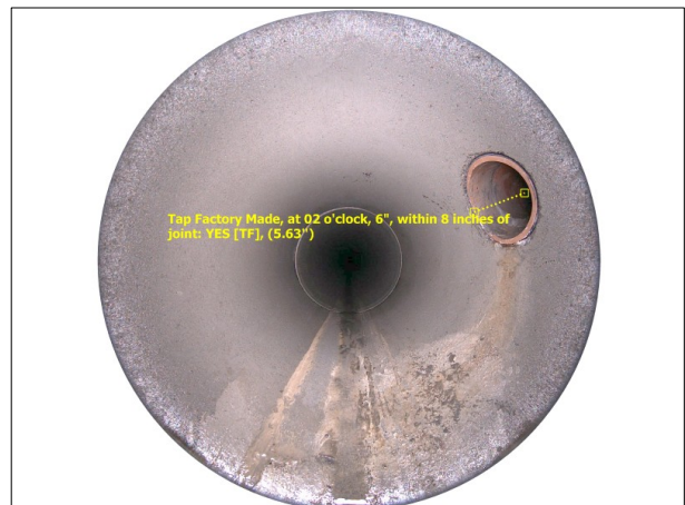
Photo: 7_4B, Media No.: 010208_1 105.97FT, Tap Factory Made, at 02 o'clock, 6", within 8 inches of joint: YES
