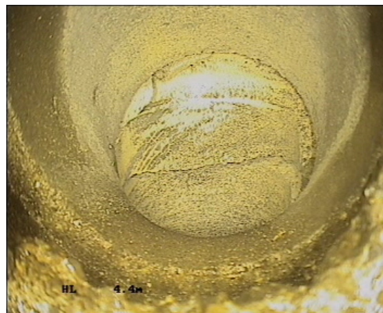
Photo: 8_2B, Media No.: 010208_1, 00:00:00 11.4FT, Tap Break-In Active, at 12 o'clock, 5", within 8 inches of joint: YES
