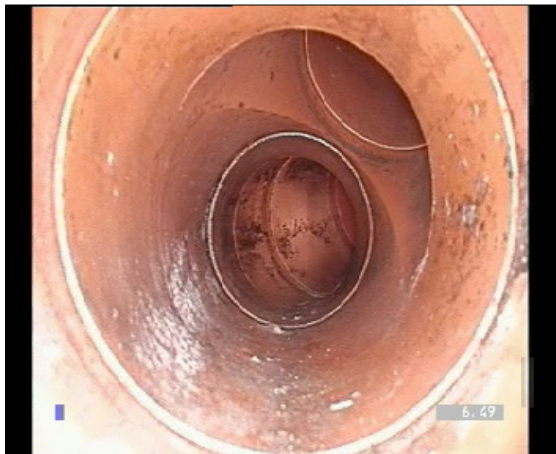
Photo: 4_3A, VCR No.: 010208_1 20FT, Tap Saddle, at 02 o'clock, 5", within 8 inches of joint: NO
