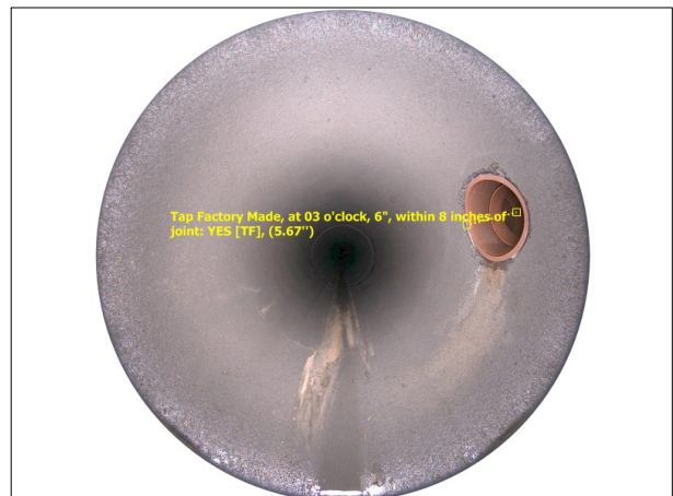
Photo: 7_8B, Media No.: 010208_1 186.42FT, Tap Factory Made, at 03 o'clock, 6", within 8 inches of joint: YES
