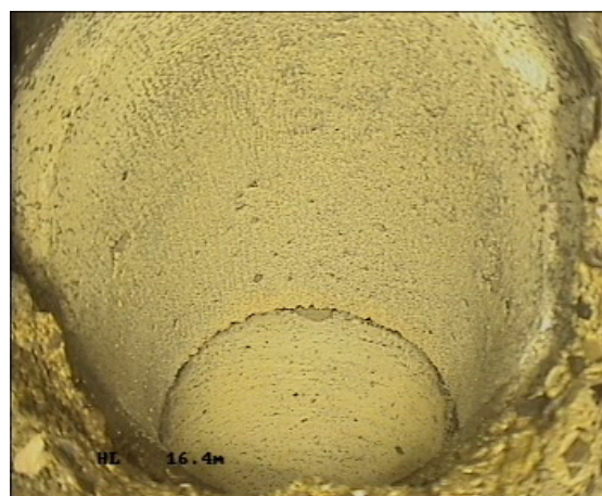
Photo: 8_5B, Media No.: 010208_1, 00:04:20 48FT, Tap Break-In Active, at 12 o'clock, 5", within 8 inches of joint: YES
