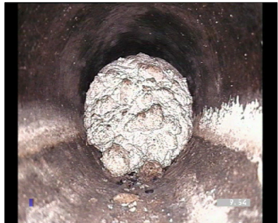
Photo: 4_6B, VCR No.: 010208_1 30FT, Obstacles Other, 100 %of cross sectional area, from 12 to 12 o'clock
