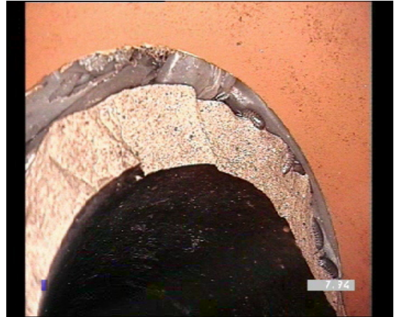
Photo: 4_4B, VCR No.: 010208_1 24FT, Vermin Other, quantity: 2 cm, within 8 inches of joint: NO / cannot be determined
